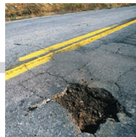
POTHOLES/ DAMAGED PAVEMENT
